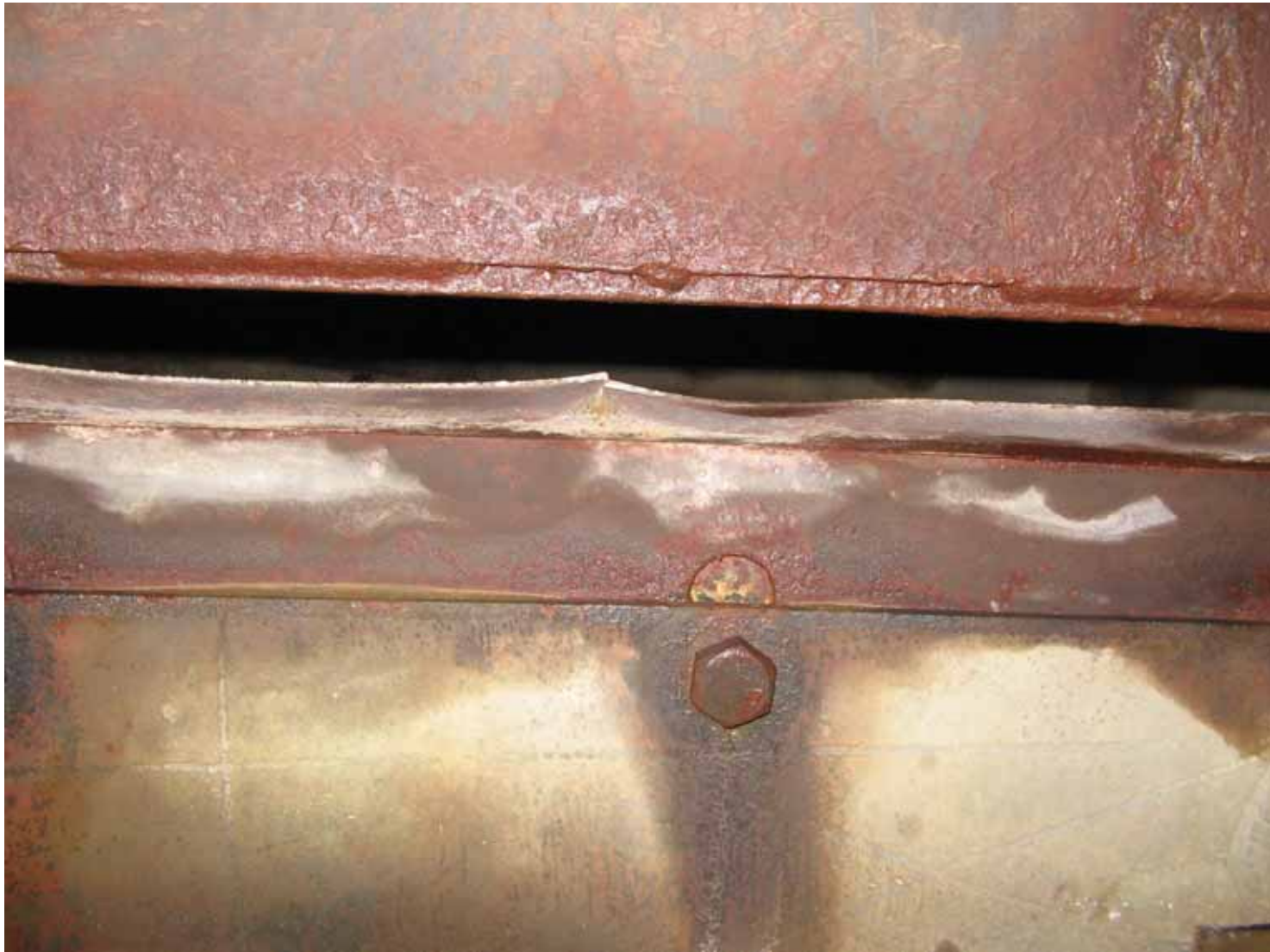
GAPS BETWEEN STANDARD RADIAL SEALS (DAMAGED) AND SECTOR PLATE
